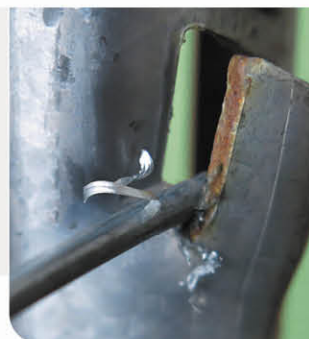
✗ Scraping of the Zn/Alu protection of the wire
